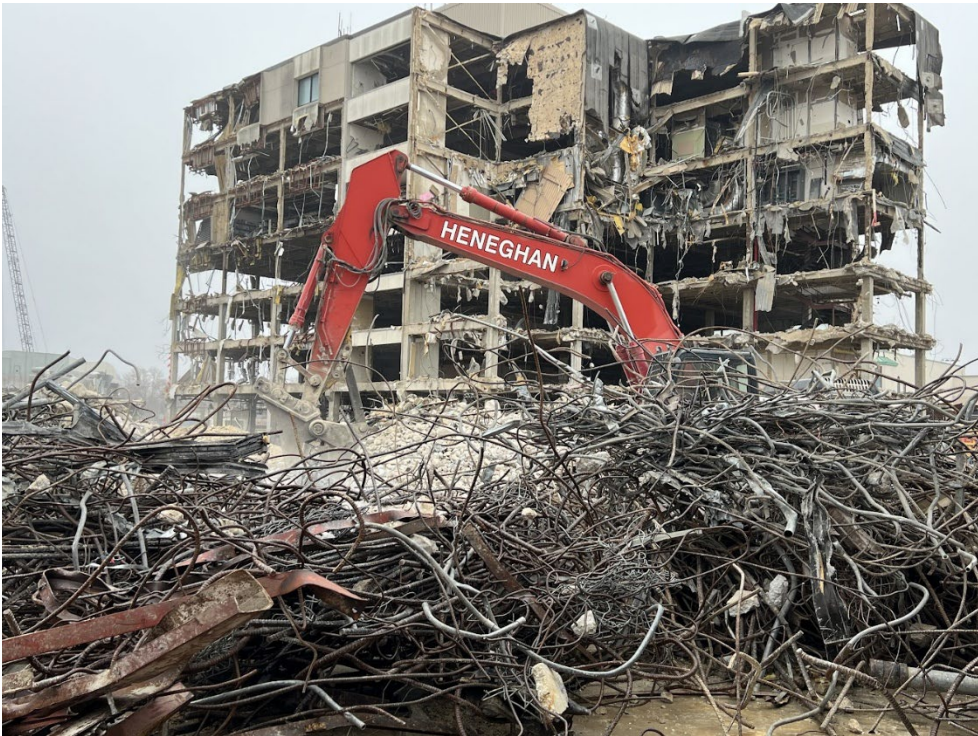
Photo-2: Rebar separated from crushed concrete
