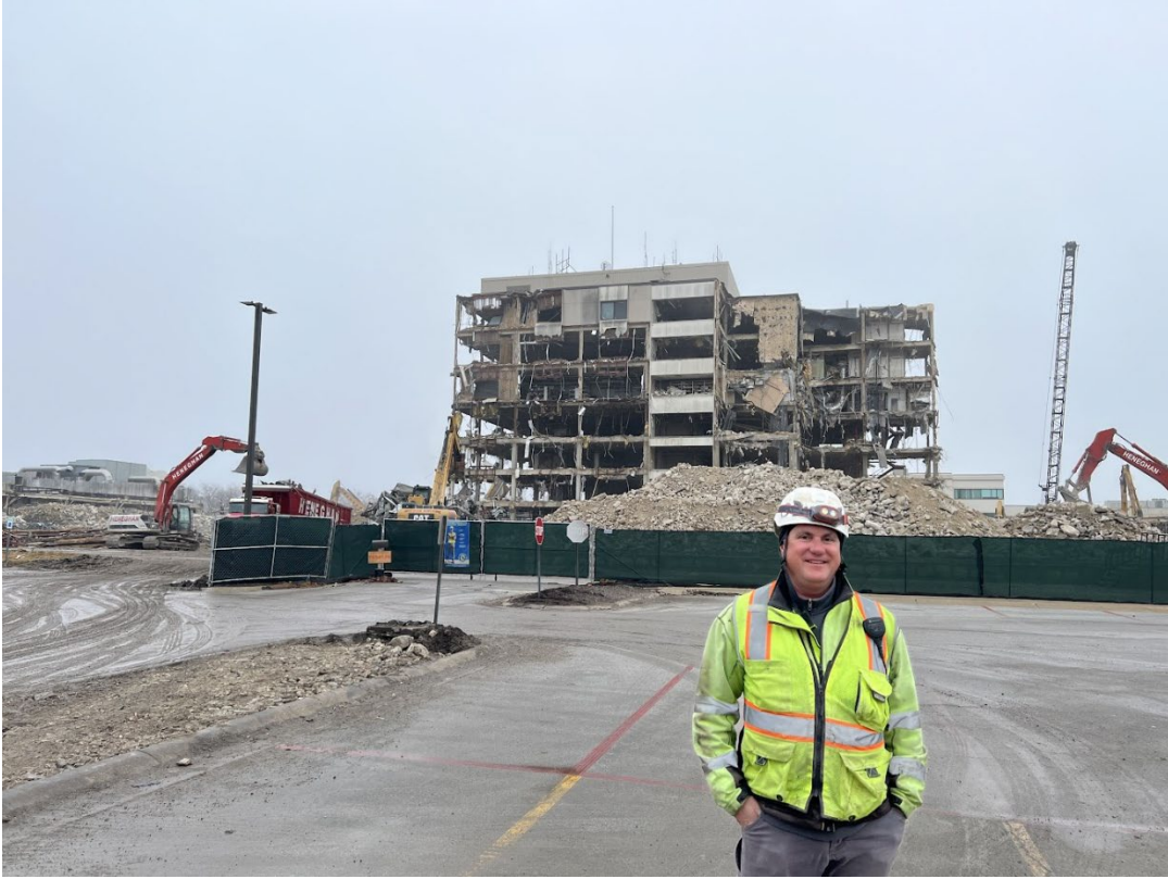
Photo-1: Andy Piano, Project Manager, Heneghan, in front of the demolition Site in Crown Point, IN
